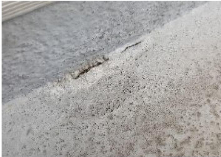
Crack On Membrane Blister
