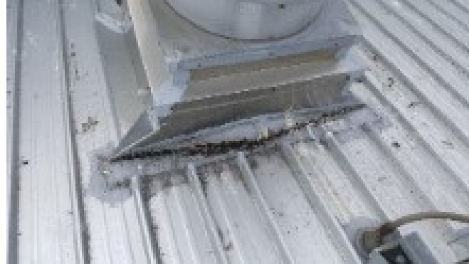
Metal Roof - Exhaust Fans
