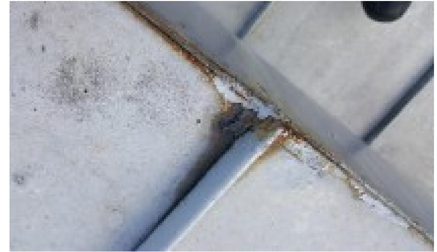
Metal Roof Rusted Copings
