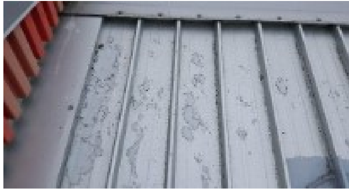
Sawtooth Metal Roof – Rust Stains
