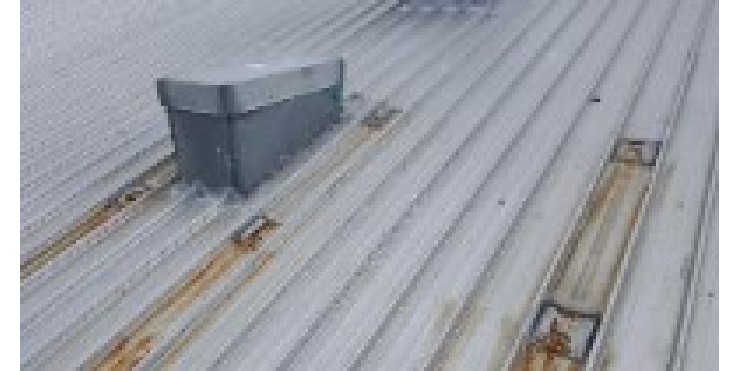
Metal Roof – Rust Stains
