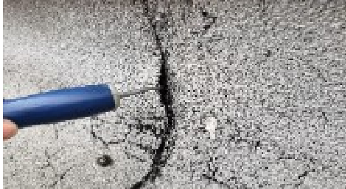
Low Slope Roof – Open Seam
