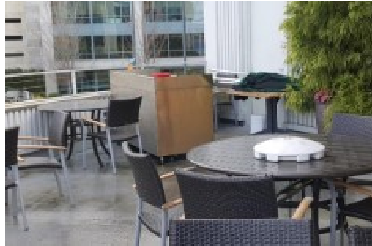
Worn Exterior Deck Membrane
